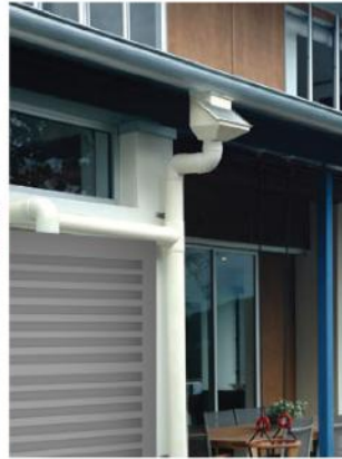
Rain Harvesting System
