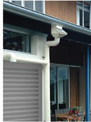
Rain Harvesting System
