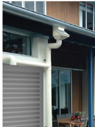
Rain Harvesting System
