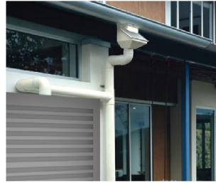
Rain Harvesting System
